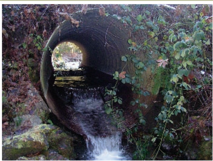
An old culvert at Gravel Creek: This culvert acts as a barrier for fish migrating upstream as the fish are forced to jump up and into the culvert to pass through.
