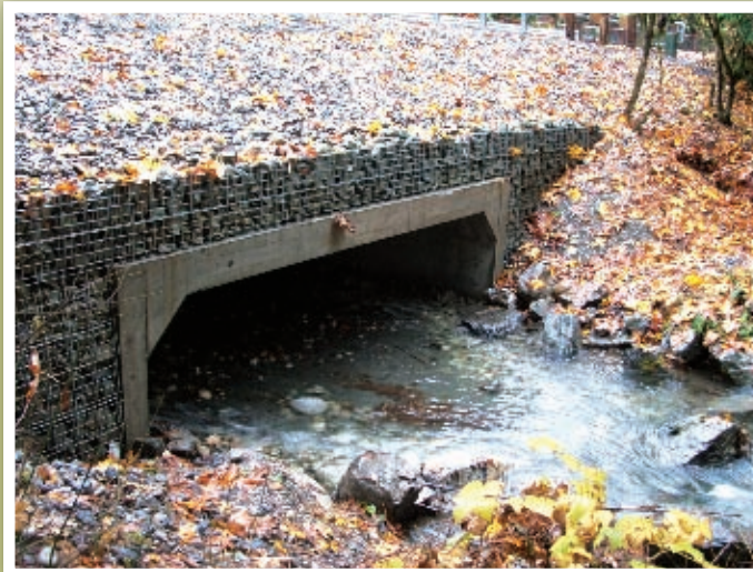
A new culvert at Gravel Creek: This culvert allows fish to swim upstream easily. It is also able to manage the flow of water that may come with rising water levels.
